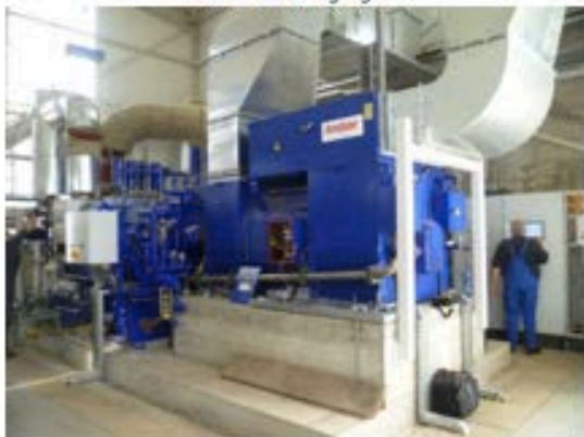
Set turbine i agregata
