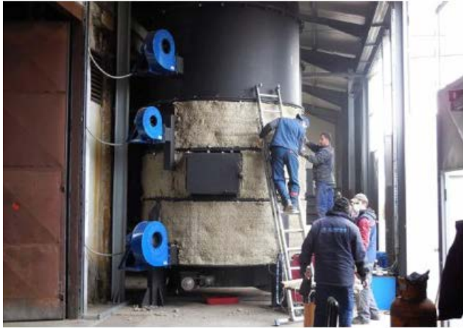
Facility for wood chips preparation
