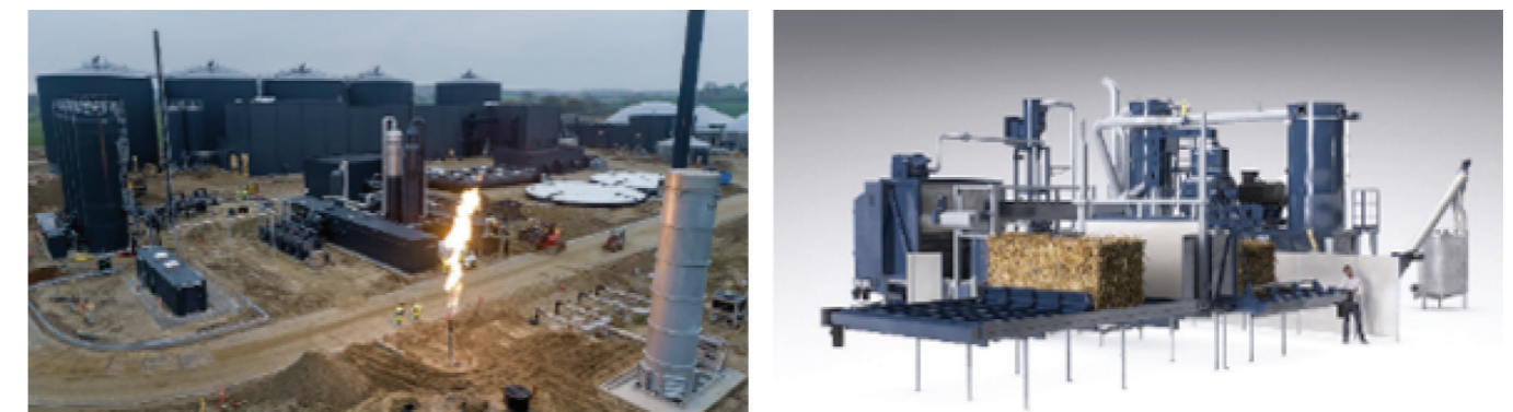
Fig. 9.9 – Biogas plant in Kværs: general view (left) and LinKa straw pretreatment line (right)
