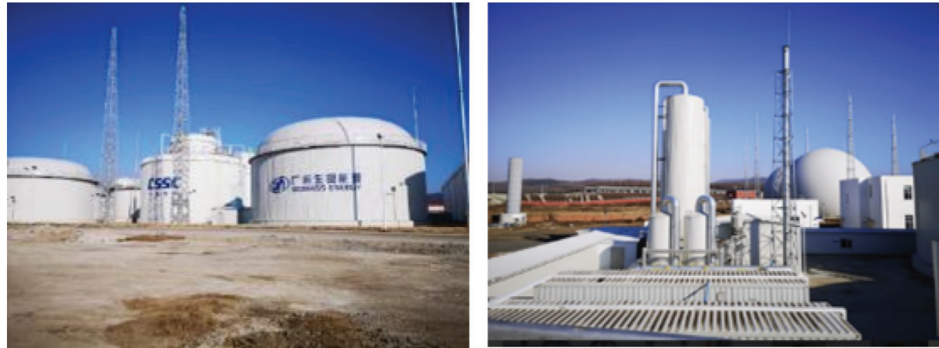
Fig. 9.7 – Harbin straw biomethane plant
