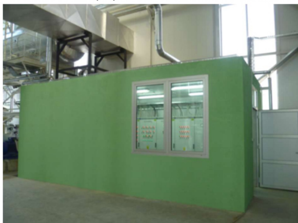
Electrical equipment for boiler control
