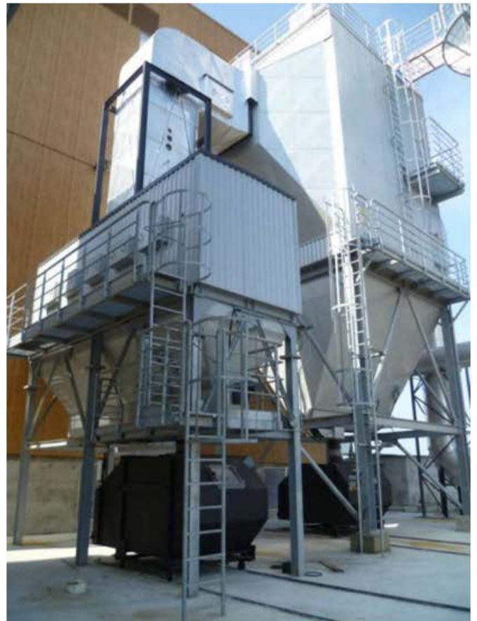
Multi-cyclone and filter
