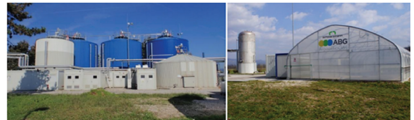
Fig. 7.1 - Photo of the AlgaeBioGas demonstration centre in Slovenia, implemented at an operating biogas plant.
