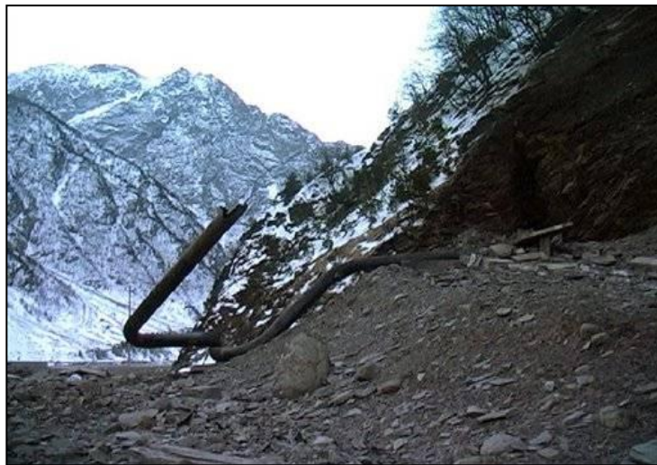
Figure 13 Damaged Section of the Vladikavkaz-Tbilisi 700 mm Gas Pipeline on Russian Territory
