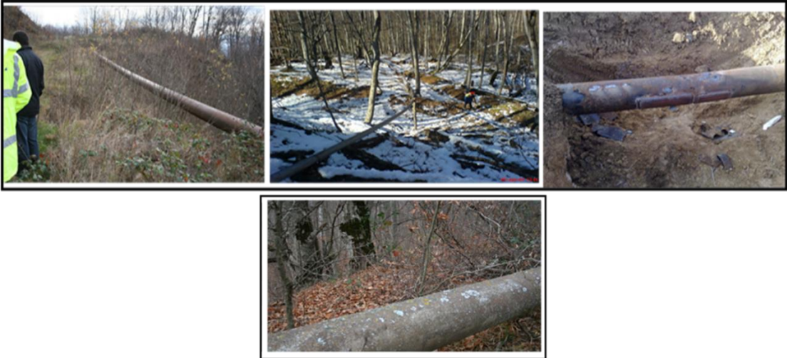
Figure 14 Kakheti Branch. Sections located in areas covered by forest and shrubland (prior to the completion of clearing work)
