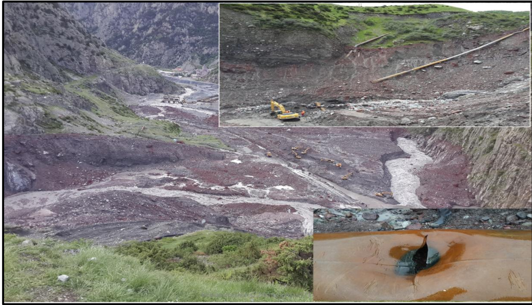
Figure 11 Sections of the main gas pipelines damaged by debris flows triggered by storm precipitation in the Devdoraki Gorge 108 (May, 2014)
