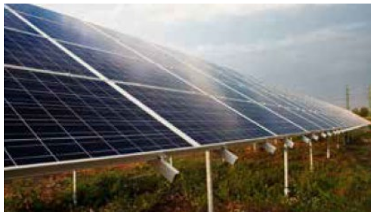
Construction of a 100 MW photovoltaic power plant on former ash dump fields at Kosovo A thermal power plant
