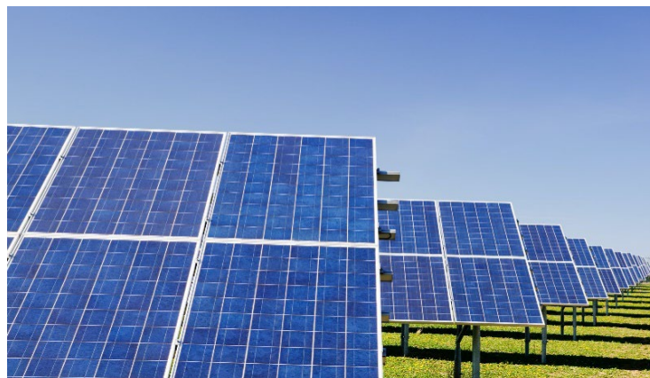
Construction of 30 MW Oslomaj 2 and Bitola photovoltaic power plants in North Macedonia
