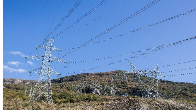
Construction of 38.7 km of transmission and distribution lines and substations in the Southeast Region of North Macedonia
