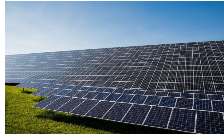
Installation of a 50 MW ground-mounted solar photovoltaic power plant in the Belsh area, Albania
