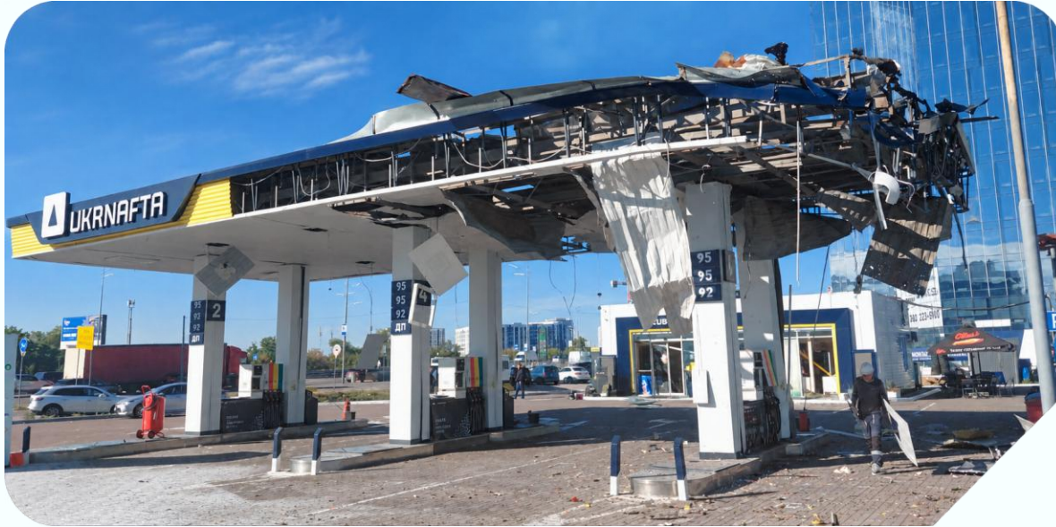
Damage: shattered windows and a damaged facade and canopy
