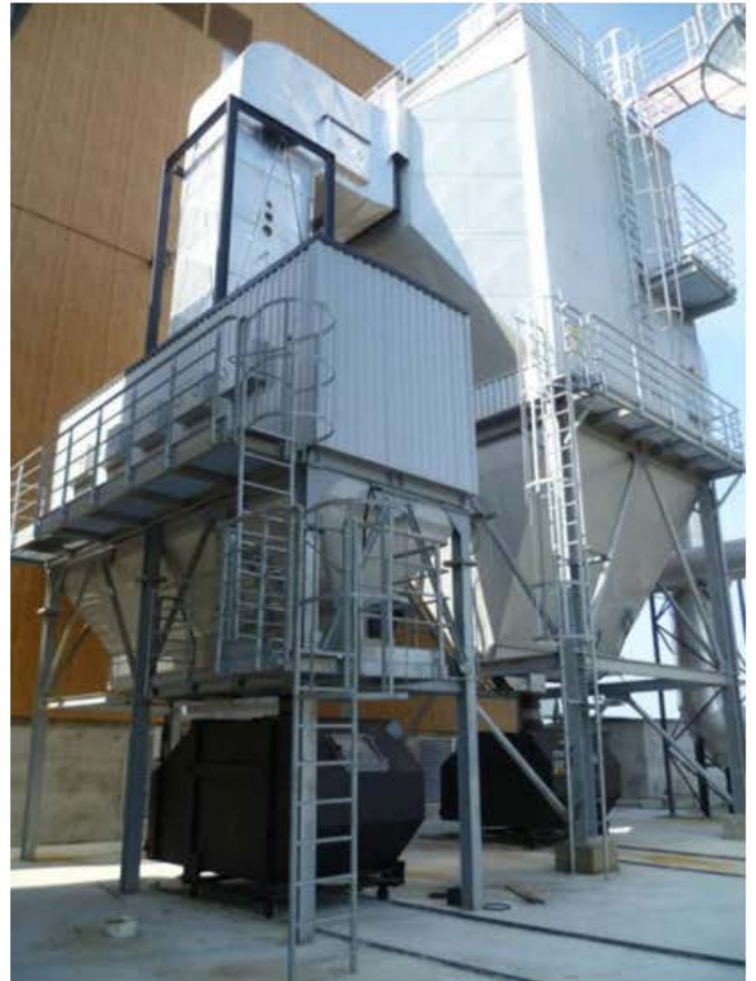
Multi-cyclone and filter
