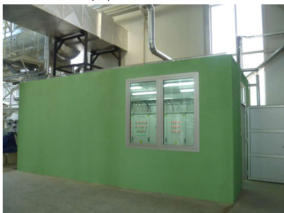
Electrical equipment for boiler control
