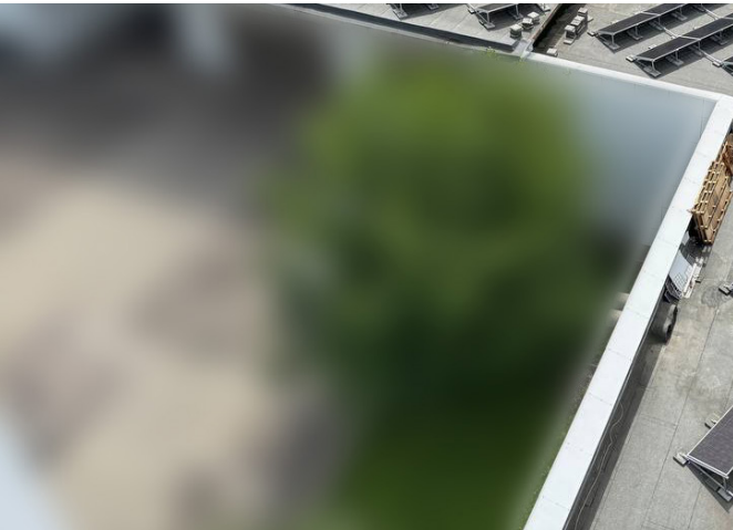
Solar panels installed as part of the Ray of Hope initiative on the roof of a Ukrainian healthcare facility.
