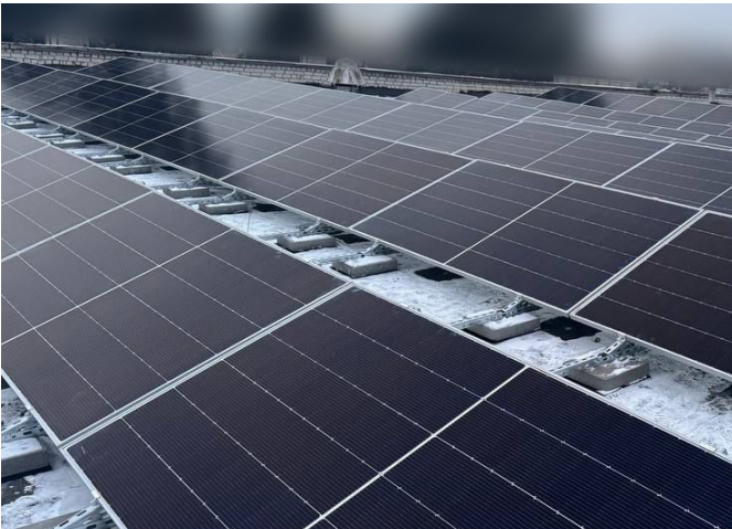
Solar panels installed as part of the Ray of Hope initiative on the roof of a Ukrainian healthcare facility.
