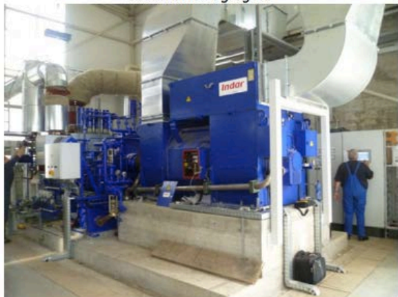
Set turbine i agregata
