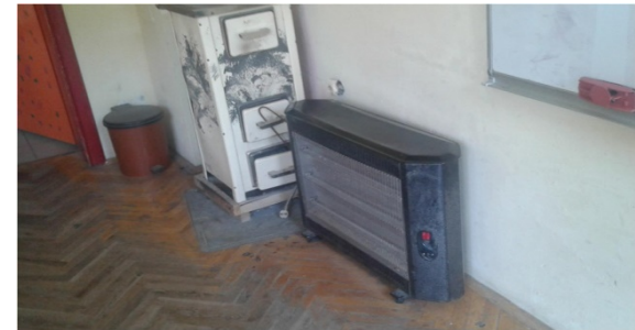
Heating appliances in Teuta School, Grashtice Village
