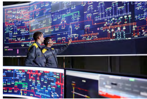
Figure 88: Videowall at dispatching center
